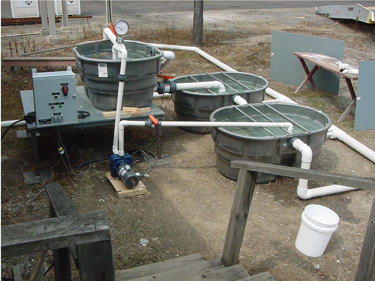
Figure 5. Trial set up on Lake Ontario, Rochester, NY. Tank 1 is the water collection tank on the platform, and contains the filter box. Tank 2, the right front tank, receives the filtered water. Tank 3, in the back, is the control tank receiving unfiltered lake water
